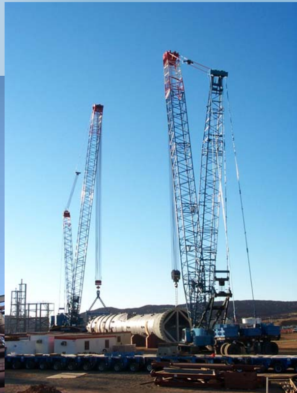
Below: Dual lift with M2250 Max-Er and M18000 Max-er preparing to up-end a column.
